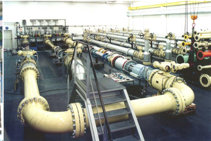
Picture of the test room of pigsar in Dorsten
