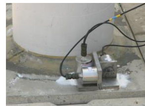
Sensors on the viaduct and pole
